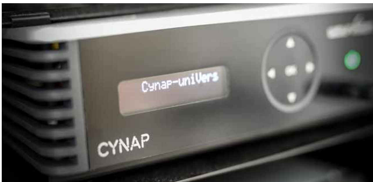
Cynap System installed at uniVersa Insurance
