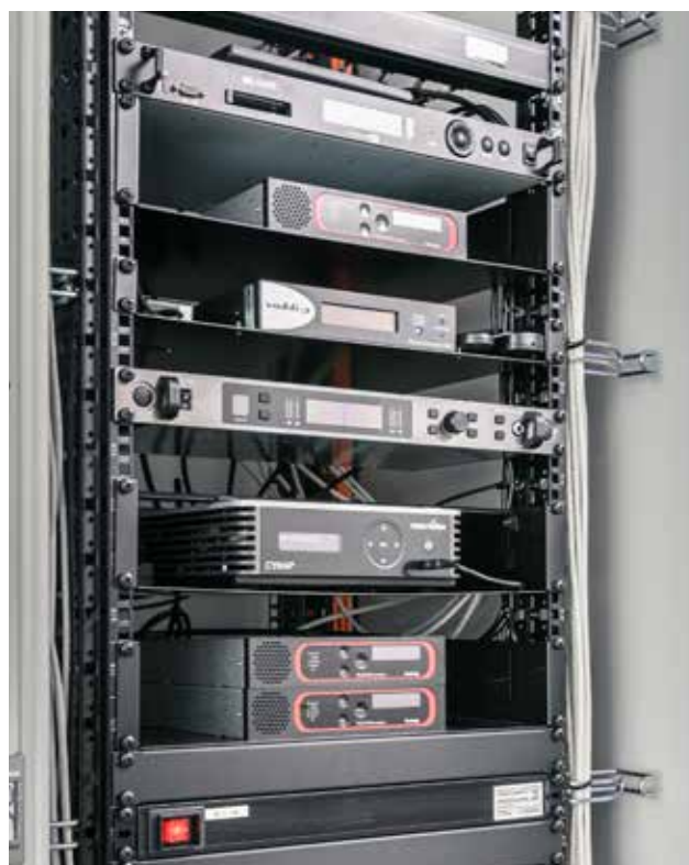
Rackmount installation of the Cynap system.
